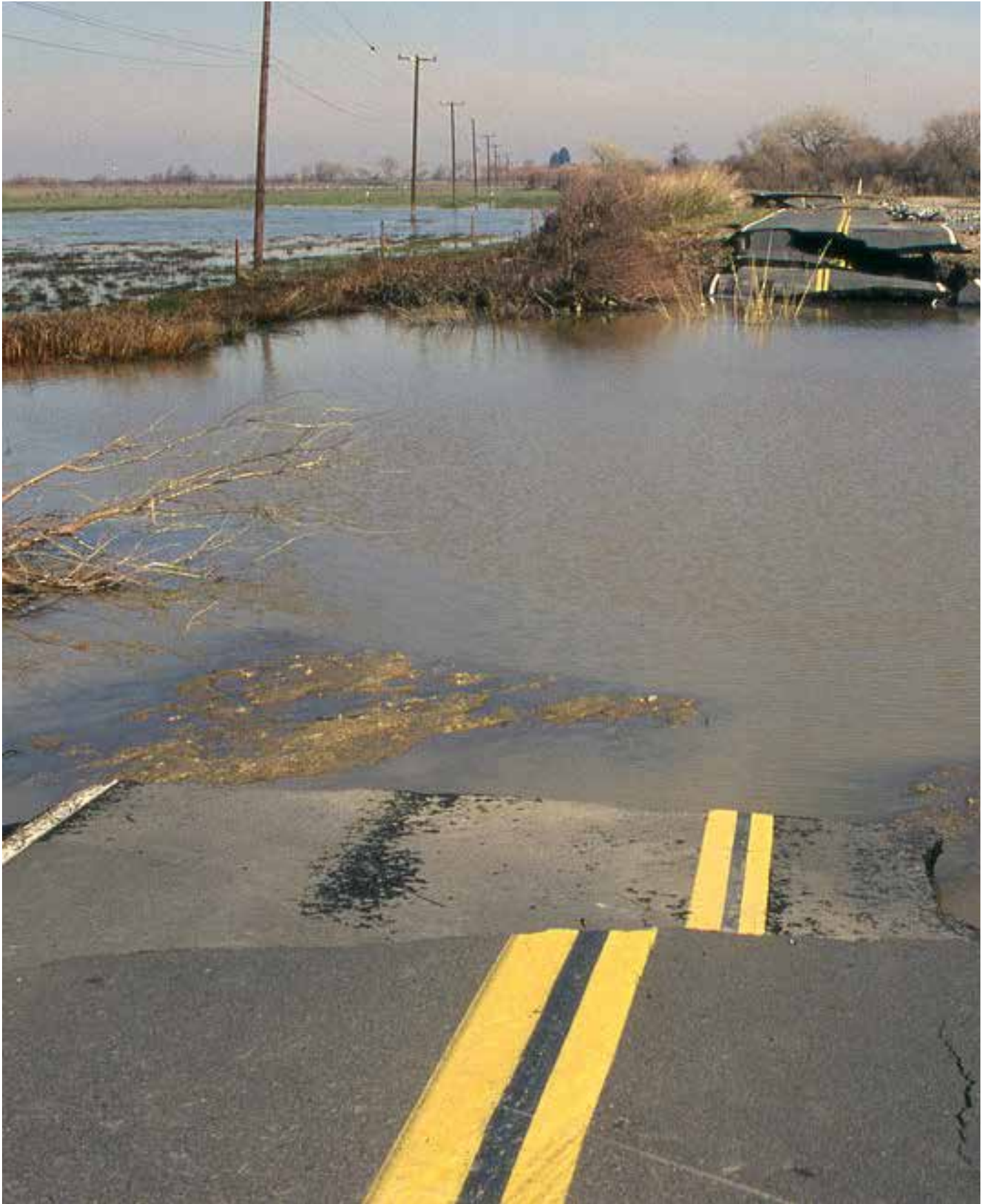
A levee breach near Rio Vista, CA. Source: US Army Corps of Engineers
